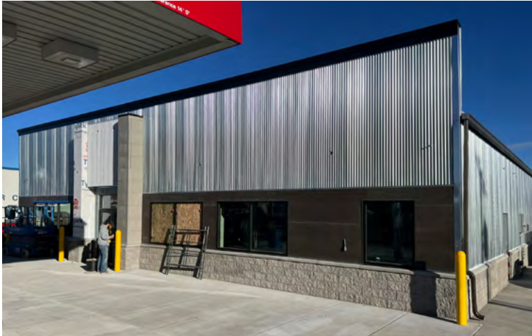
The exterior is almost done! Our signs should be installed in the next two weeks. Luckily most of the outside work got done before the cold weather hit.
