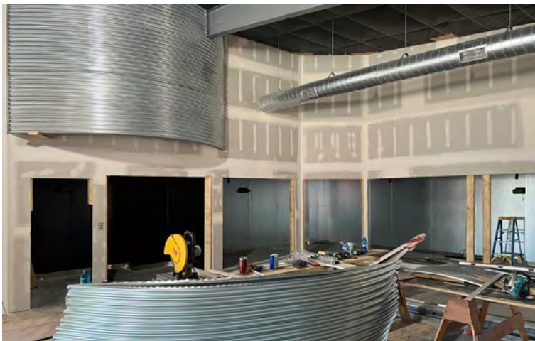
Work is progressing rapidly on the inside. The coolers are now in, and the beer bin is taking shape.
