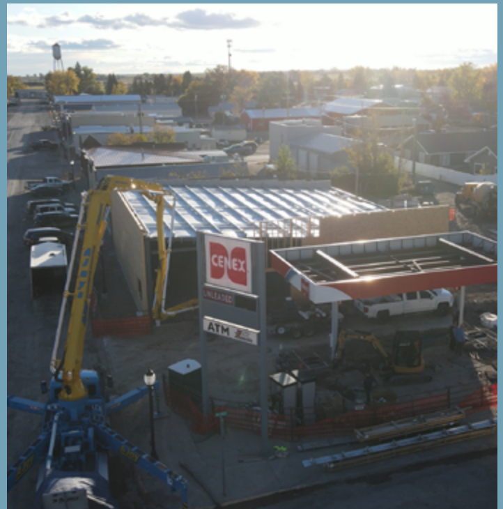
Now the walls are up and the concrete floor has been poured. It's starting to look like a store again.
