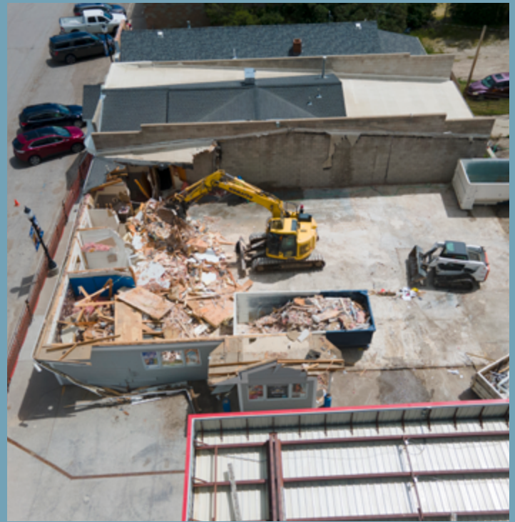
It didn't take long for an excavator to get the job done. The store was gone before July, and left a blank canvas for our new construction.
