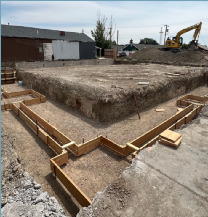
The construction crew dug down a few feet to ensure our new foundation would be on solid ground, then built frames for the new footings.
