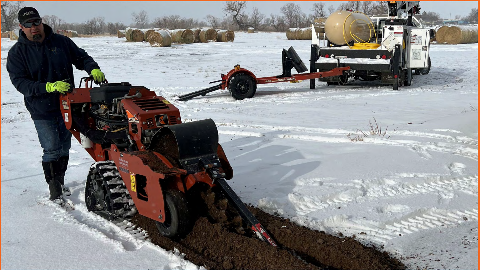
Chad Holzheimer digs a trench to bury a propane line before he sets a new tank. According to Chad, it's much harder to dig through frozen dirt, as it becomes as hard as concrete.
